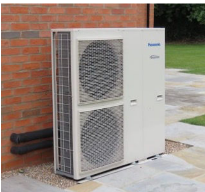
Photo 41. Air source heat pump (note the external pipework can also be visually unattractive and should be positioned carefully).
