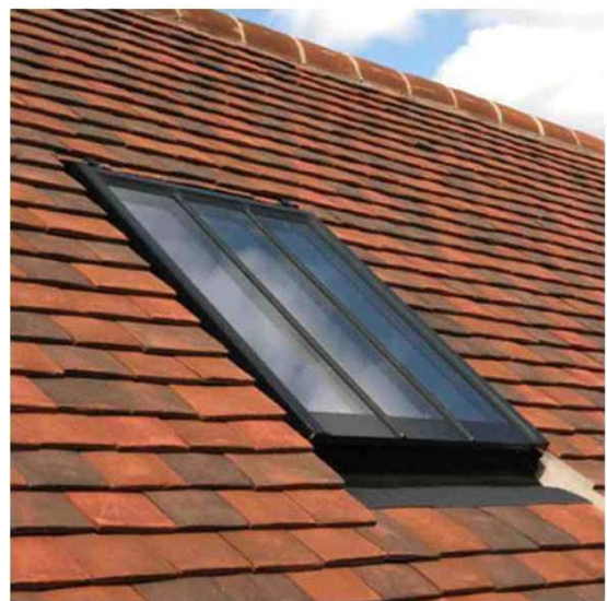
Photo 35. Conservation type skylight flush with roof surface.
