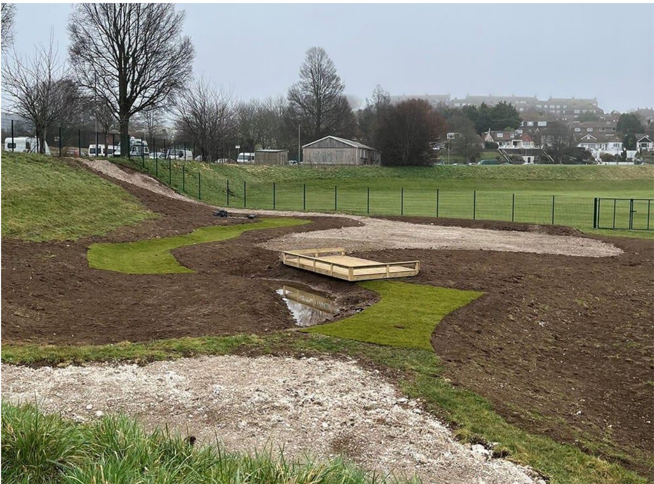
Figure 10.10 SuDS in Carden Primary School
