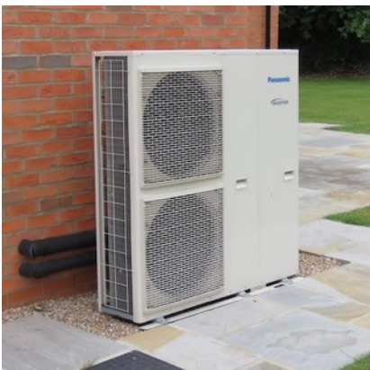
Photo 41. Air source heat pump (note the external pipework can also be visually unattractive and should be positioned carefully).
