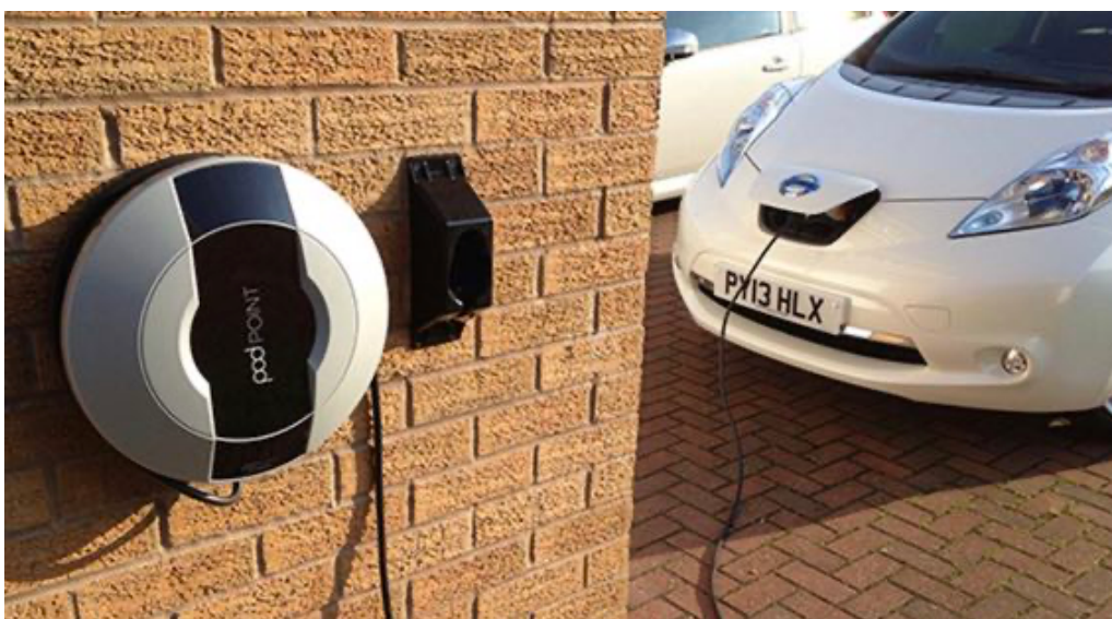
Photo 43. EV charger is less intrusive on a side wall.
