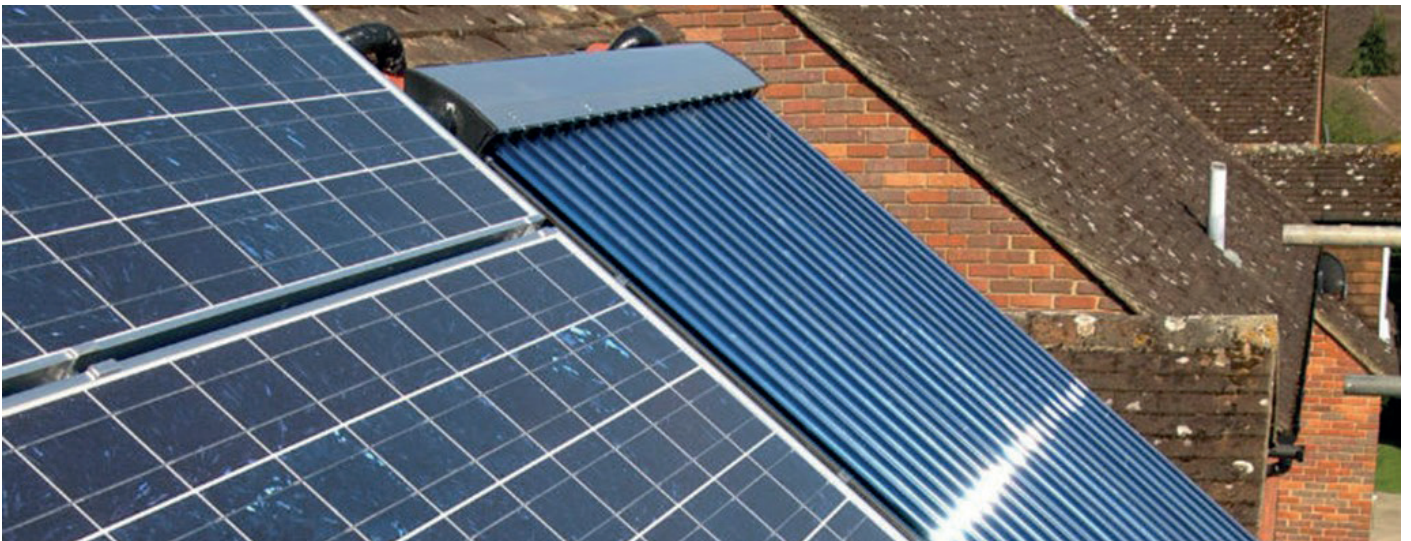
Solar photovoltaic panels (left) and solar thermal panels (right)
