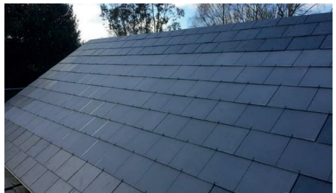
Low visual impact PV tiles on a slate roof
