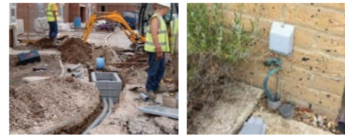
Figure 8.19: (left) Laying ducting (BT Openreach) with inspection chamber and (right) duct end with drawstring to allow for future easy laying of fibre cable to a house.
