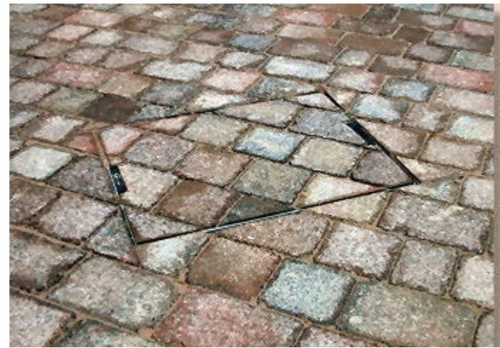
Figure 8.17: Service manhole recessed cover helps to protect integrity of paving, even when at an angle. ( Pavingexpert.com ).
