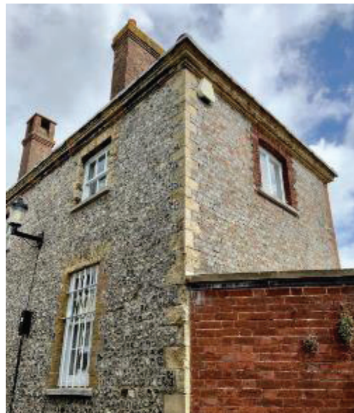
Figure 12.2: Galleted flint and stone quoins, red brick are used on a building in Lewes.
