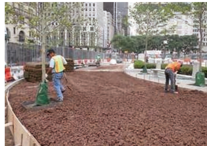
Figure 9.17: An example of a structural soil system (clean stone lattice with soil added) in New York City (CU-Structural Soil).
