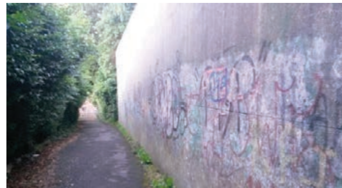
Figure 7.17: Places in built up areas that are not overlooked are more at risk from vandalism.
