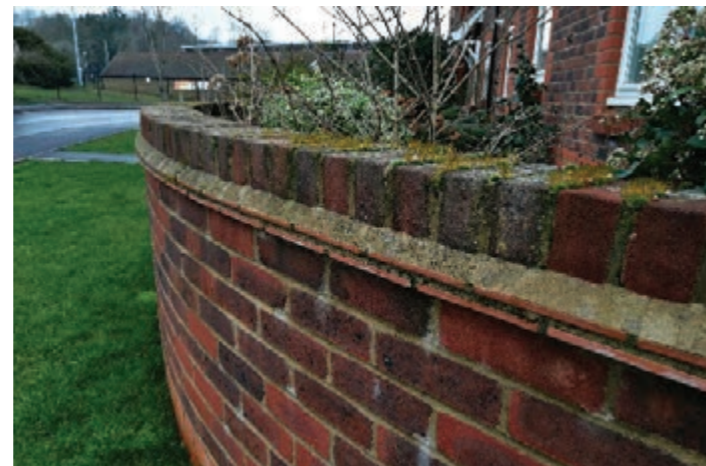
Figure 12.8: Traditional tile creasing in brick wall coping detail, in modern Midhurst development.
