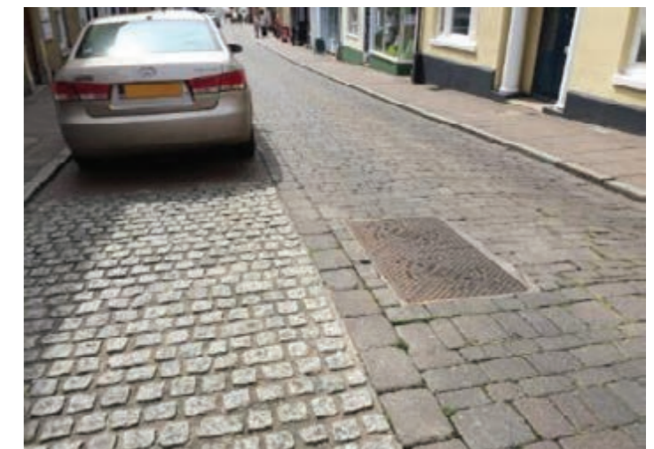
Figure 8.1: Instead of ugly white or yellow lines, parking places can be indicated by a change of road surface.
