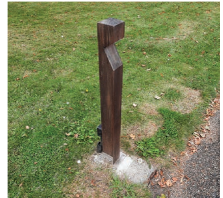
Figure 8.20: Simple timber bollard lighting directing light downwards in West Dean Estate.
