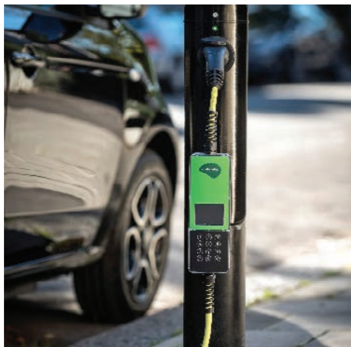
Figure 8.28: A converted lamp post housing an on street EV charge point (Lucy Zodian).
