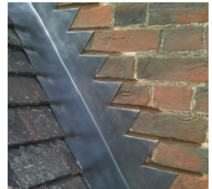
Figure 12.30: Good quality flashings in a roof junction.
