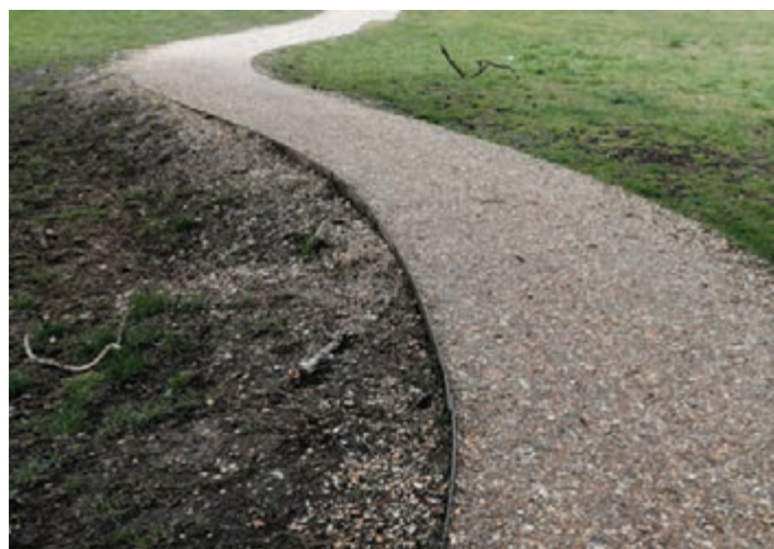
Figure 12.52: Steel edge details can also describe elegant curves in a subtle way and are more robust and long lasting than timber. Compacted stone footpath in Hampshire park.
