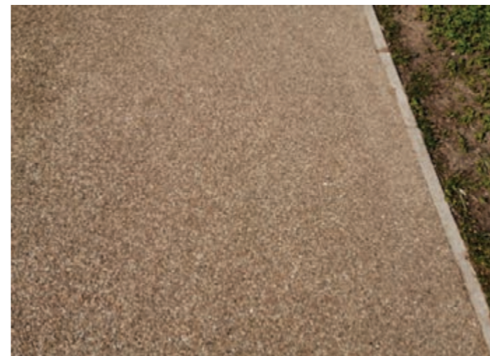
Figure 12.57: Resin bound aggregate footpath.
