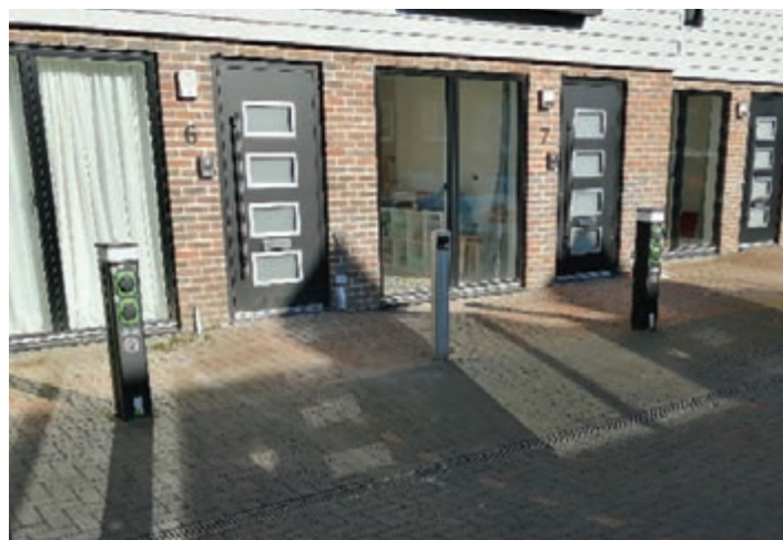
Figure 8.29: EV charge points serving residents in a town house development in Lewes and also serving as traffic bollards.
