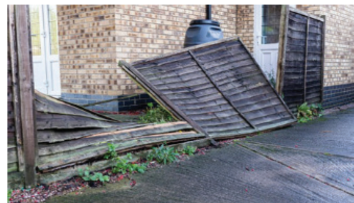
Figure 11.2: Poor quality and lightweight timber panel fences are not a good long-term solution in the public realm as they are not very robust.
