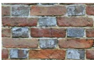
Photo 30. Brickwork in Flemish bond with red brick stretchers and grey/blue burnt headers seen on Upham Church and the Manor House
