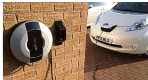
Photo 41. EV charger is less intrusive on a side wall.
