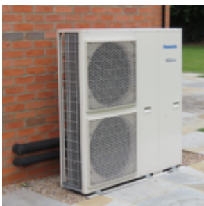
Photo 39. Air source heat pump (note the external pipework can also be visually unattractive and should be positioned carefully)
