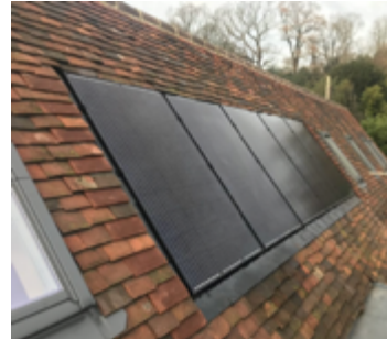
Photo 40. Solar Photovoltaic panels in a regular pattern and recessed into roof tiles.
