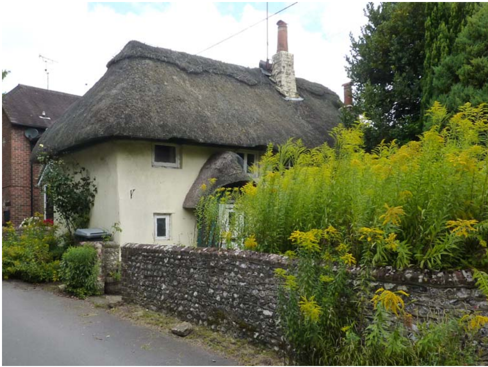
Figure 28: Sunrise ; an important survival of cob construction within the village and a building identified as ‘vulnerable’ in the National Park’s Buildings at Risk Survey
