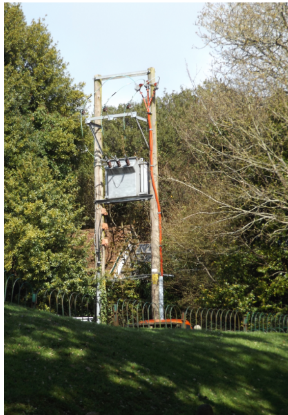
Figure 11: Other elements which detract from the Conservation Area and setting of the house include the entrance to the 'bunker' (above) and the electricity transformer (below)
