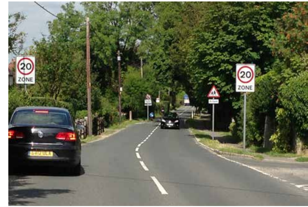
Excessive highway signing and lining - B 2116
