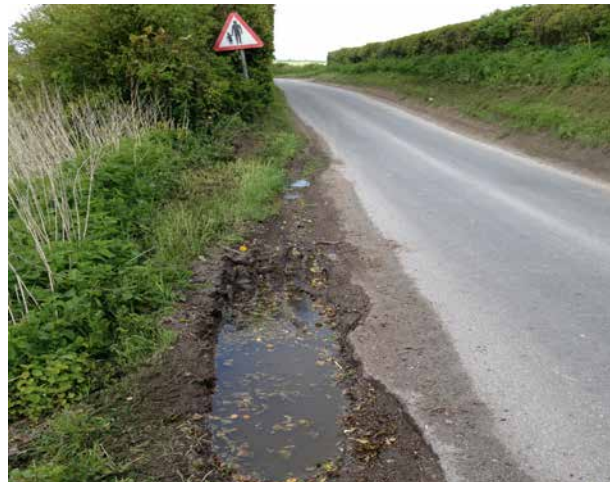
Damaged verge from poor edge detailing
